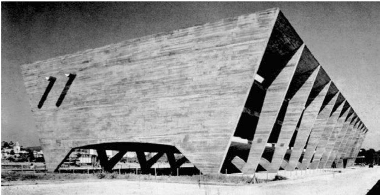
Figure 3.3: Museum of Modern Art, Rio de Janeiro, by Affonso Eduardo Reidy, 1948 (construction site picture).
