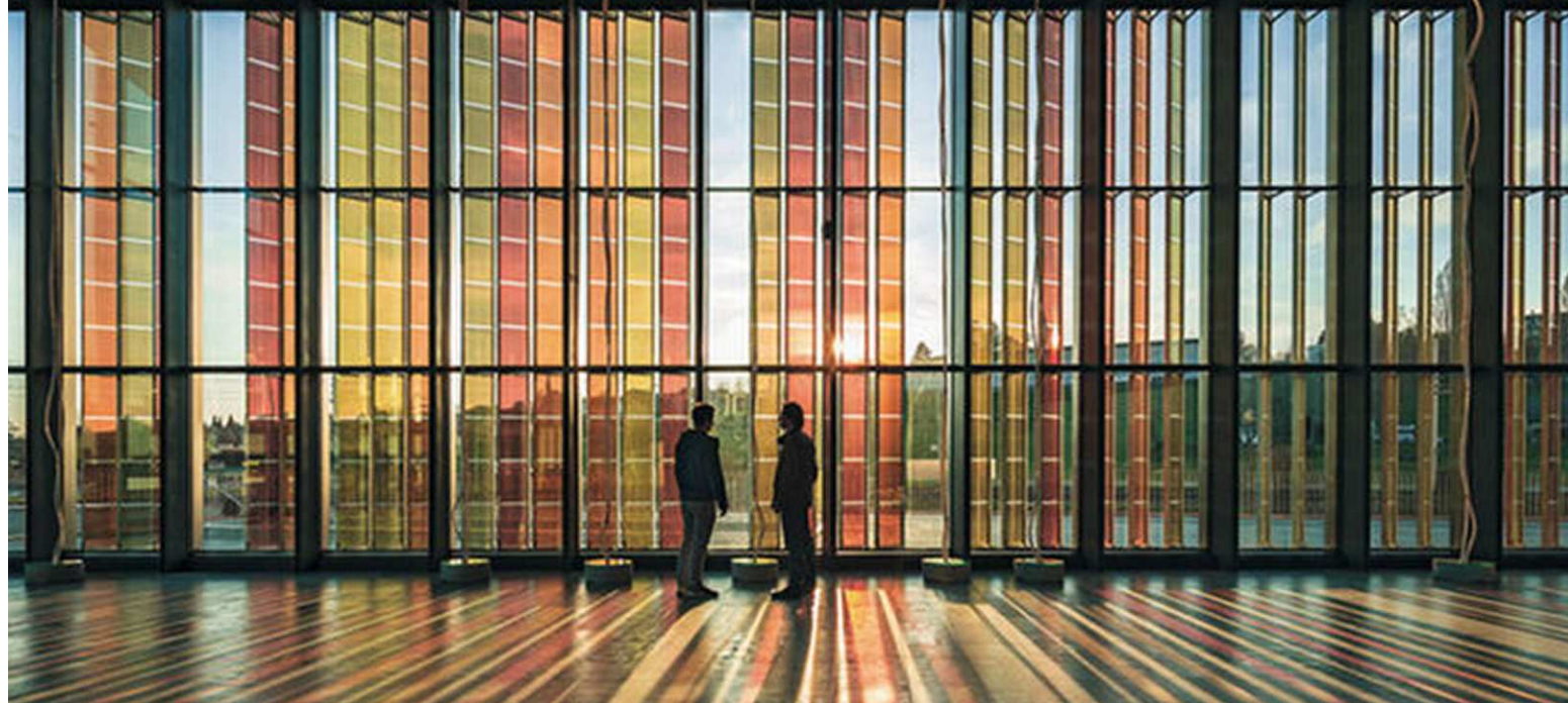
Fig. 24 – Sunscreen of the EPFL QUARTIER NORD SwissTech Convention Center Retail and Student Housing (Richter Dabl Rocha & Associés, 2014, Ecublens, Switzerland) made with DSSCs device.
