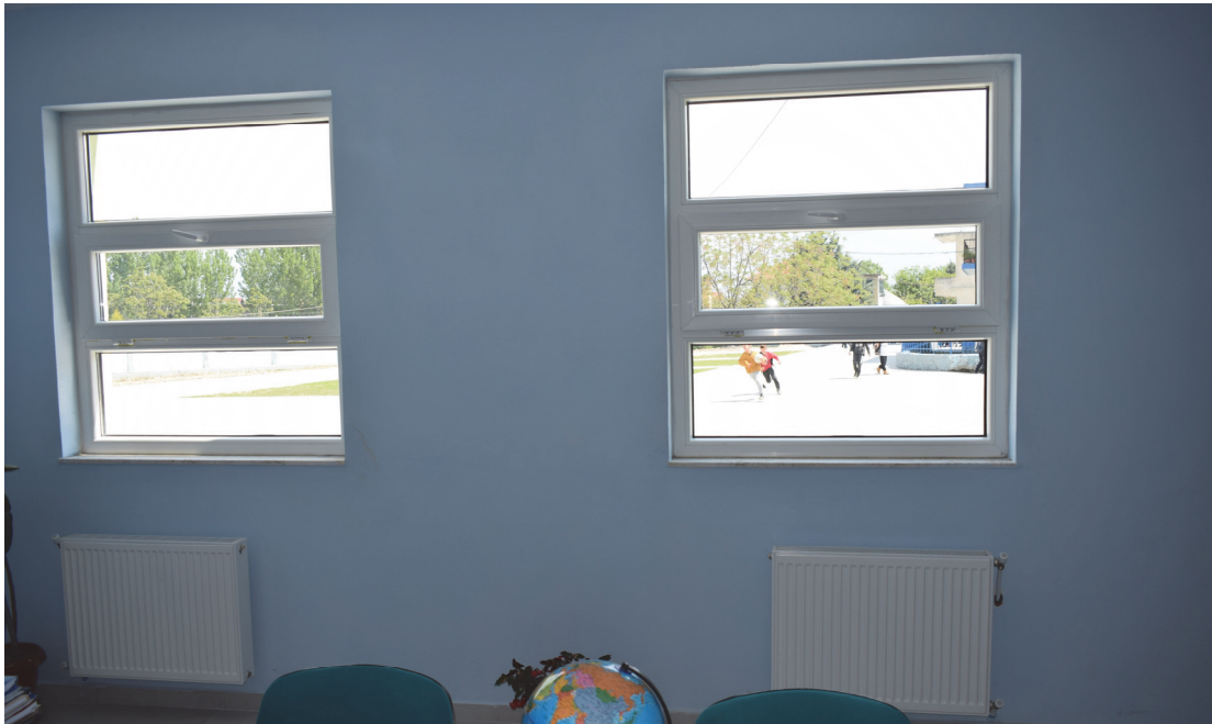
Figure 24 Radiators in the renovated school "Nene Tereza" in Laknas, Kamza Municipality- source the Author
