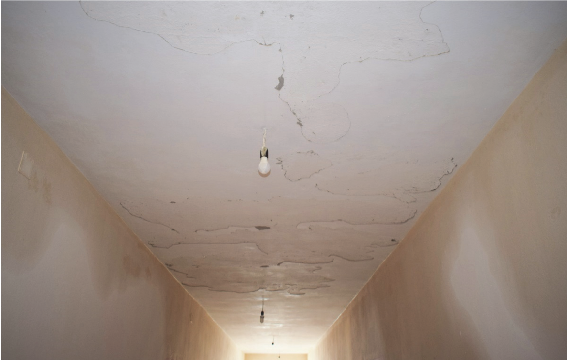
Figure 32 Degradation in the interior and exterior of the school – source: the Author
