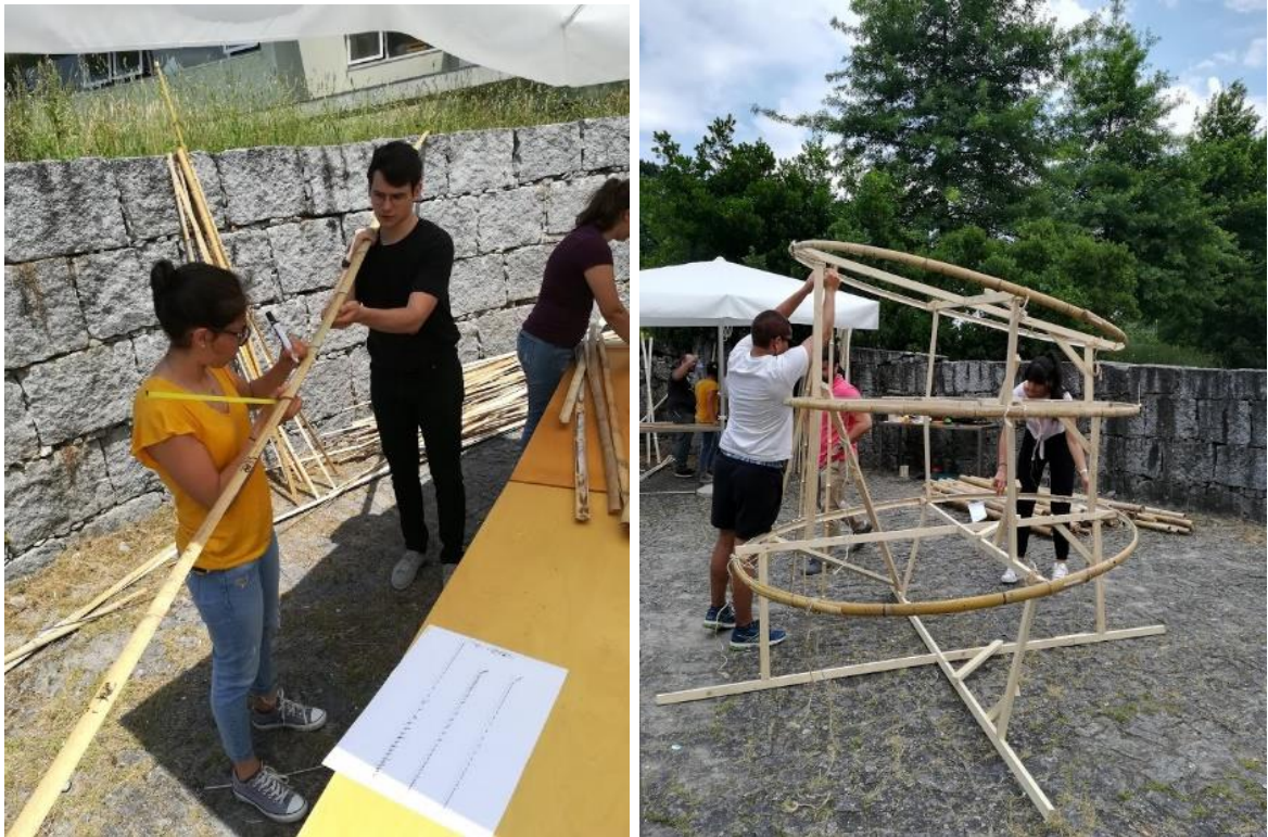
Figure 90 (a) Marking the horizontal structure for the connections (b) assembly of the first part photo: author (2018)
