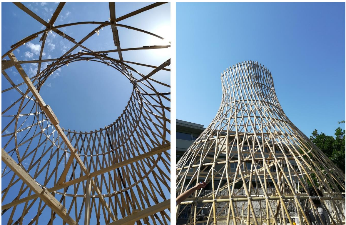
Figure 93 View from the inner part with guide structure visible (a) view from the outer part (b). Photo: author (2018)
