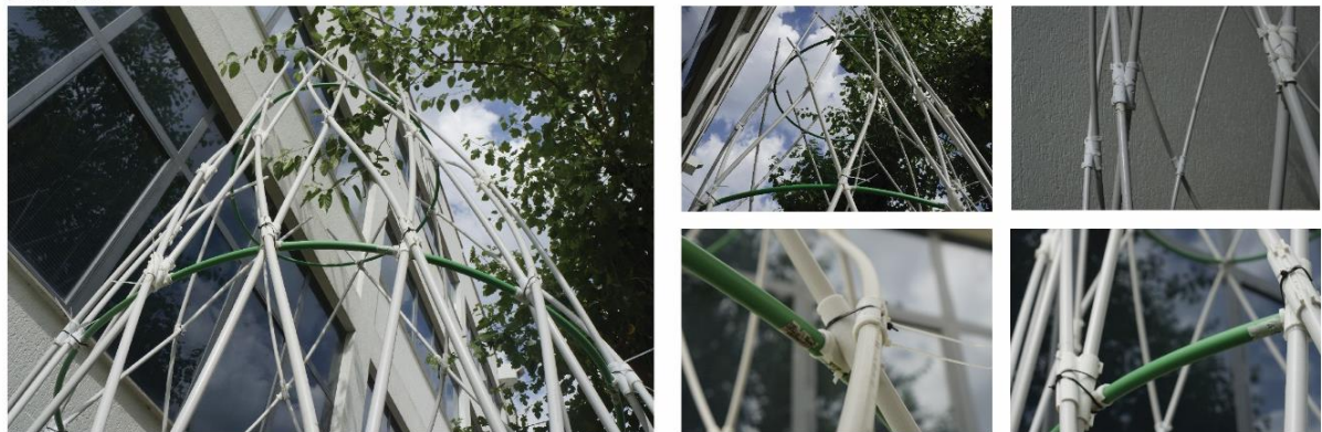
Figure 107 Assembly process of the PVC pipe structure and details. Photos: Author and Sara Codarin
