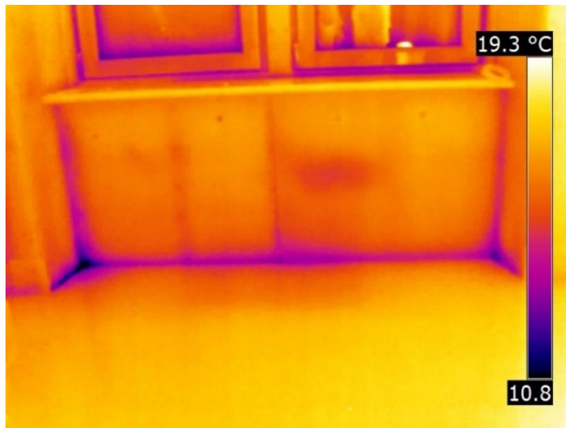
FIGURE 22 - INFRARED IMAGES OF THE TEST ROOM
