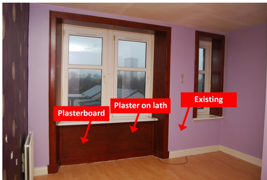
FIGURE 14 - EXTERIOR WALL IN THE DEMONSTRATION ROOM, PRIOR TO PREPARATORY AND RETROFIT WORKS, WITH PROPOSED WALL FINISHED INDICATED IN RED, REPLACING THE EXISTING PLY BOARD
