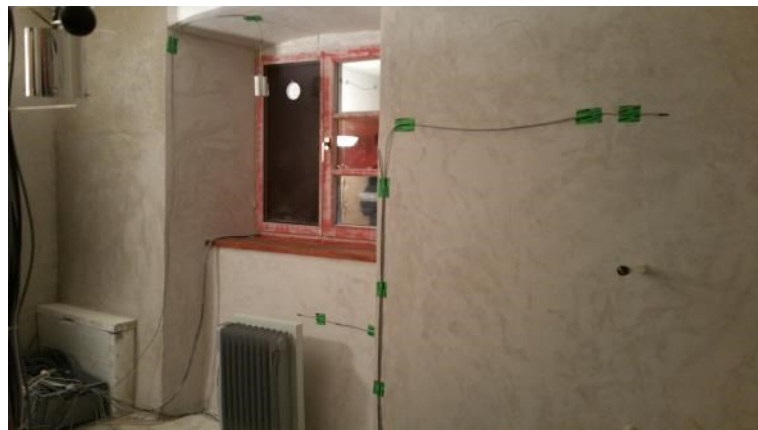
FIGURE 30 - SENSOR SET UP ON THE INNER SURFACE AFTER THE APPLICATION OF THE MORTAR (IMAGE COURTESY OF FRAUNHOFER)
