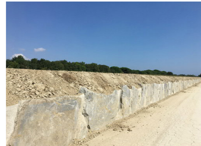
Fig. 107. Ravenna (Italy). Construction site of the right bank of the Bevanella canal by the Romagna Reclamation Consortium. The embankment increases protection from hydraulic risk, in an area where it is already high and also increasing due to climate change effects. In depressed areas it is necessary to regulate the water flow with surface works.
