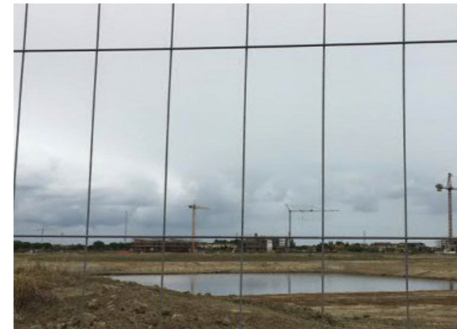
Fig. 100. Cesarea Park, Ravenna (Italy). Construction site in a urban expansion area in Ravenna, where a green zone able to maintain the hydraulic invariance following the urbanization is built. Inside the park is created a 9-meters-deep lake that allows to keep a water surface while collecting rainwater and reloading the aquifers.
