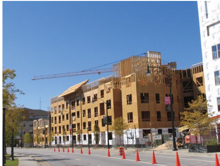
Figure 2.32 Case 8 - Exterior view; Student Housing - University of Washington Source: http://www.woodworks.org/design-and-tools/ (accessed March 12, 2017)
