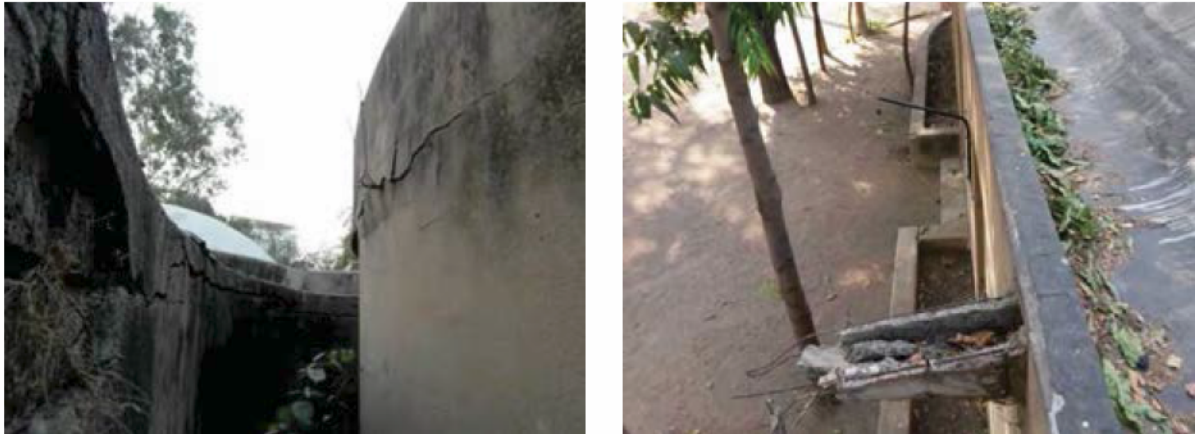
Figure 9.7: Current photograph showing building's cracking and deterioration.
