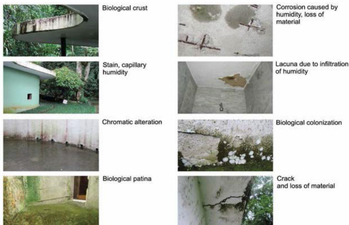
Figure 8.26: the main deterioration issues identified during the diagnostic survey.
