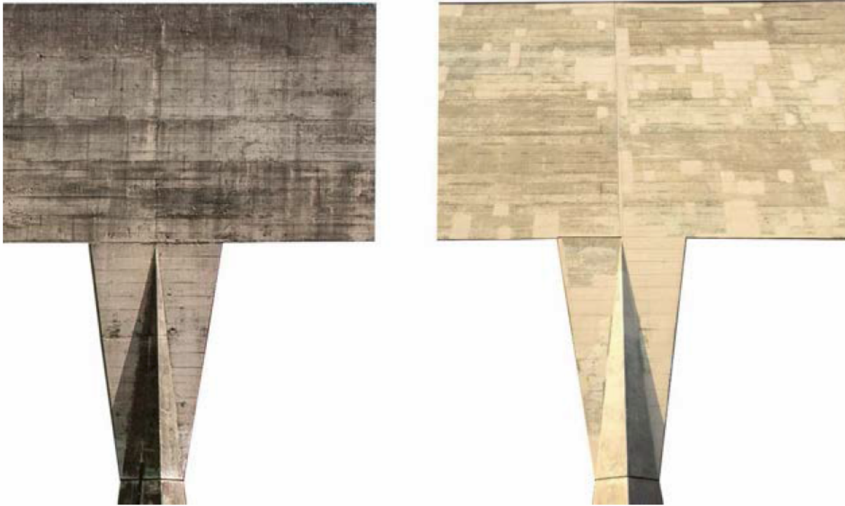
Figure 8.13: FAU USP building, one of the external pillar before (left) and after the heavy treatment in 2015.
