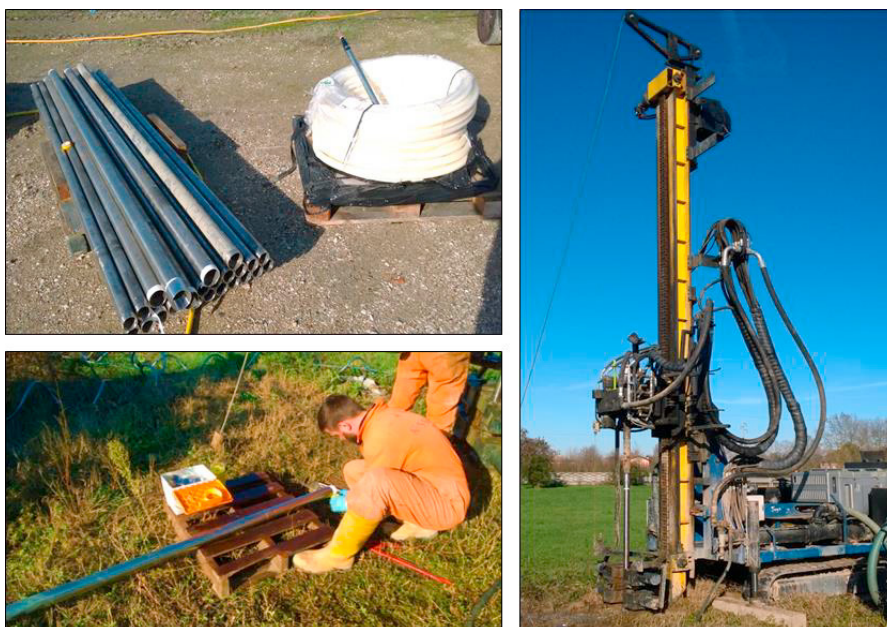
Fig. 3. Some installation phases of the newly developed Coax GSHP at the Molinella test site.
