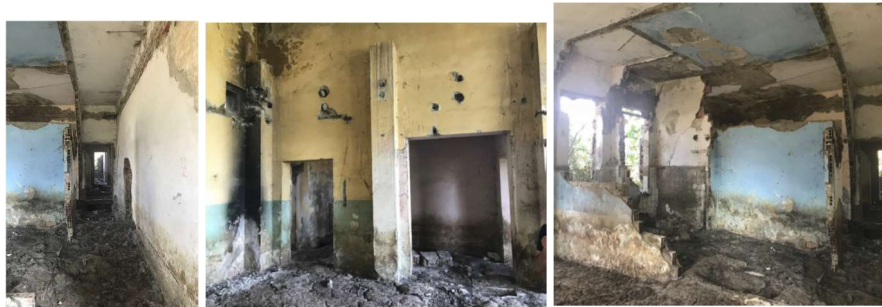
Fig. 4 Photo of the state of degradation of the interior, 2018 (source: author's)
