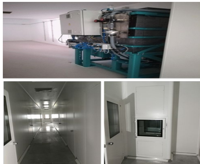
compound): (top) the first hot cell installed; (bottom left) the central laboratory lane; (bottom-right) one of the passbox between different lab areas.
