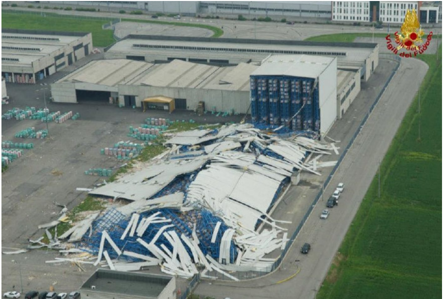
Fig. 1 Aerial view of the struck industrial area showing the collapsed warehouse (courtesy of the Italian National Fire Corps)
