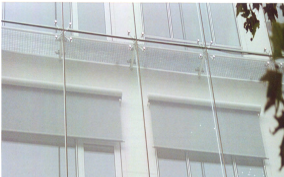
Figure 1. A fully-glazed double-skin ventilated glass façade in the refurbishment of an existing building. Torno International Headquarters in Milan (Italy)
