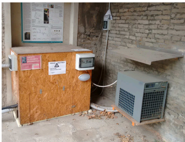
Fig. 2.4 The thermally insulated wood casing and the chiller.
