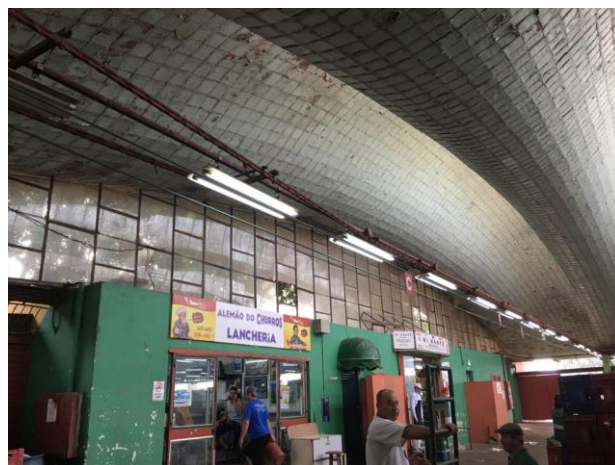
Figure 1: Gaussian Vaults of the CEASA Market, in Porto Alegre, designed and built by Eladio Dieste between 1969 and 1972.
