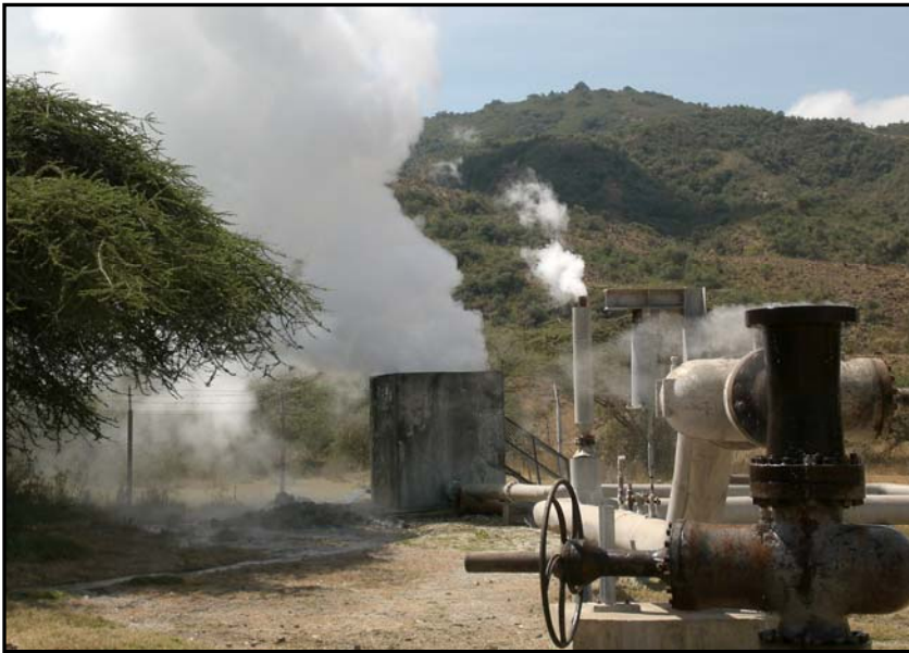
Figure 2.4: Deep (>2 kms) geothermal well at Aluto-Langano geothermal field (photo: January 2007)
