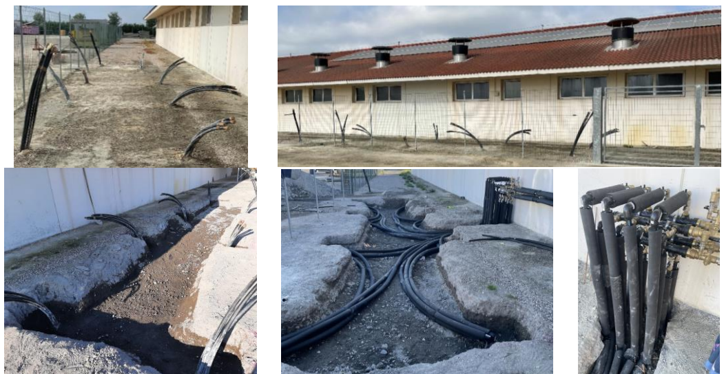
Figure 17. Realization of the BTES system: installation of the 8 BHEs and pipe connections.
