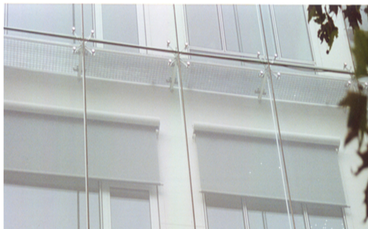
Figure 7. Double-layer glass façade in the refurbishment of a 1960s building in Milan.
