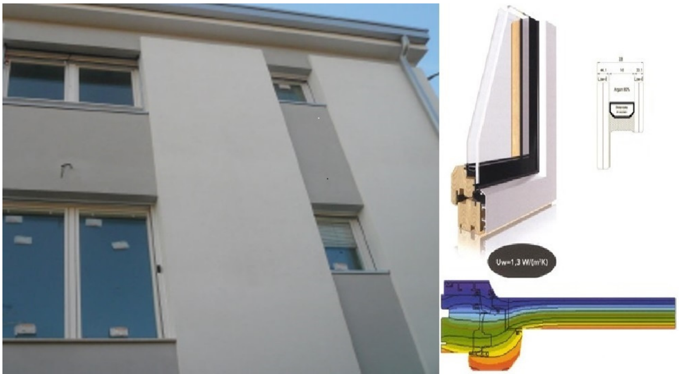
Figure 5. Replacing existing windows in a post-war building in Ferrara (Italy) with composite high-performing window frame (wood–polystyrene–aluminum) to improve the U value of the window.
