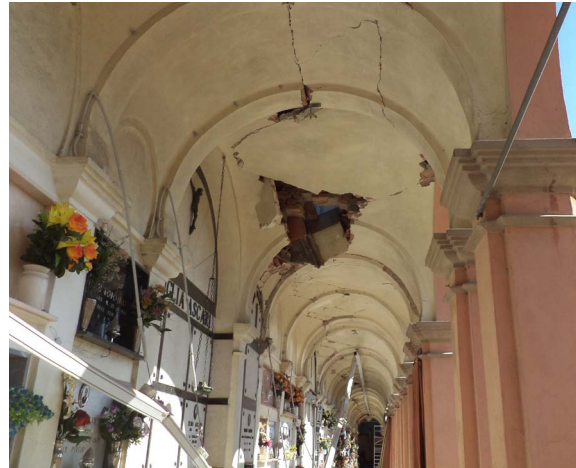
Fig. 12. Projection elements collapse. Ph Arch. Pedrini
