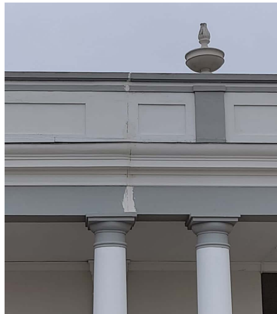
Fig.19. Mirabello cemetery in Emilia Crater area. Damage for constructive irregularities. Ph. Arch. Luca Cei
