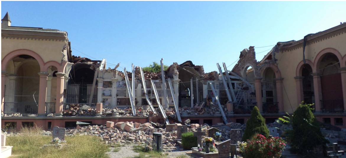
Fig.8. Collapse of a part of cemetery structure. Ph Arch. Pedrini
