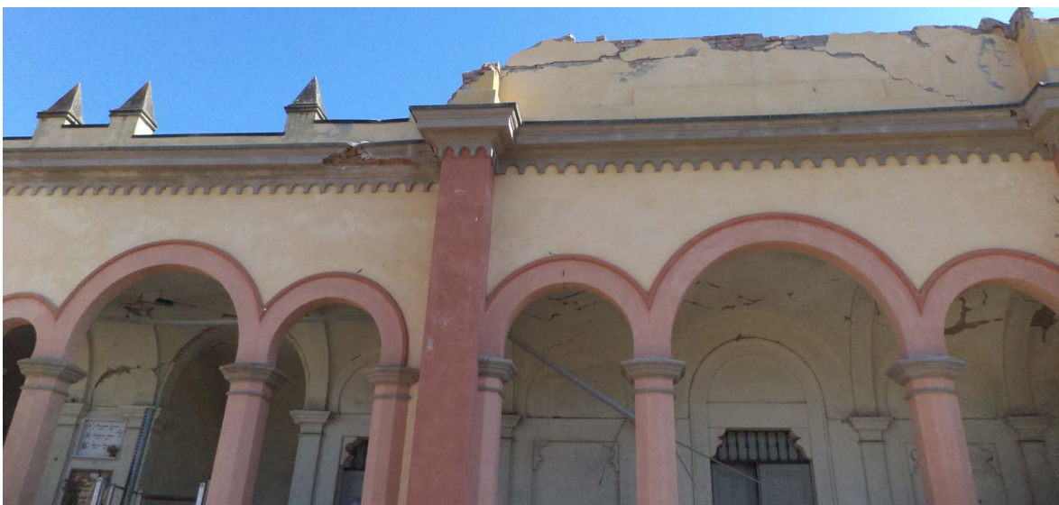
Fig. 13. Gable collapse. Ph Arch. Pedrini
