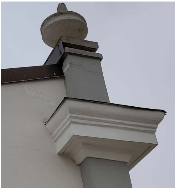
Fig.18. Mirabello cemetery in Emilia Crater area. Damage to projecting elements. Ph. Arch. Luca Cei
