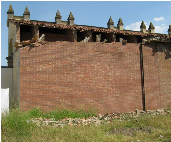
Fig. 11. Rear wall collapse. Ph Arch. Pedrini
