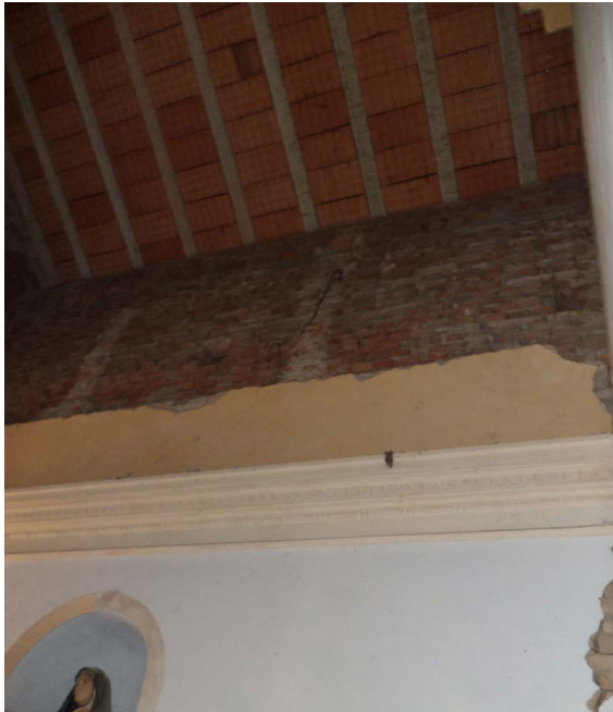
Fig.14. Damage to the vault. Ph Arch. Pedrini
