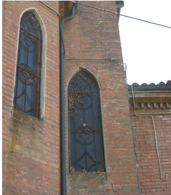
Fig.15. Shear in the apse. Ph Arch. Pedrini
