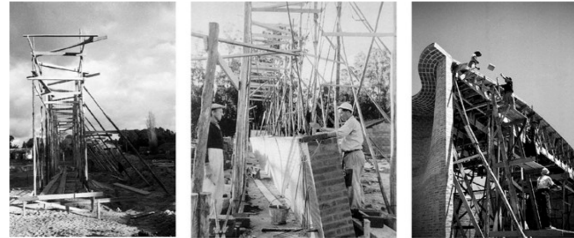
Fig. 5.19. Images of the construction site of the Church during the late fifties (Courtesy of Eladio Dieste Foundation, source: Rossato et al., 2025b).
