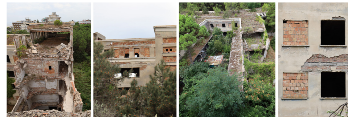
Fig. 8.17. State of conservation of the external surfaces of Former Colonia Varese.
