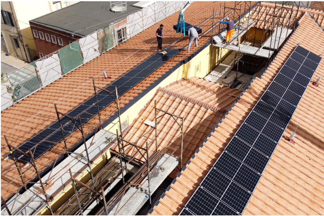
Fig. 4. Installation of the photovoltaic system on Ex Sert roof (Photo by Gianni Nucci).
