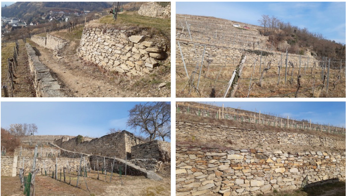
Figure 4. Details of the dry stone wall terraced area CH1 (credits to Rainer Vogler).
