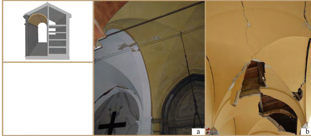
Figure 5: Cemetery of Bondeno (a) and cemetery of Mirabello - damage to the vaults
