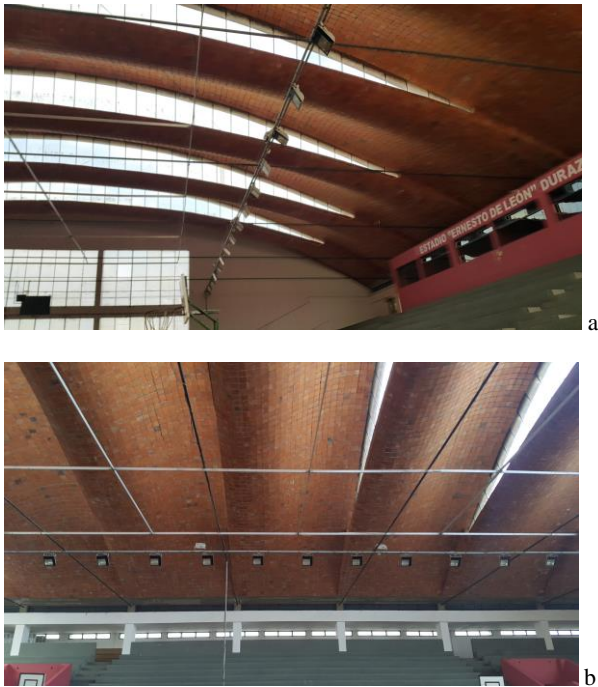
Figure 2. Transverse take (a) and longitudinal take (b) of the Discontinuous Gaussian Vaults of the Durazno Gymnasium, in Durazno (Uruguay), designed and built by Eladio Dieste between 1973 and 1975.
