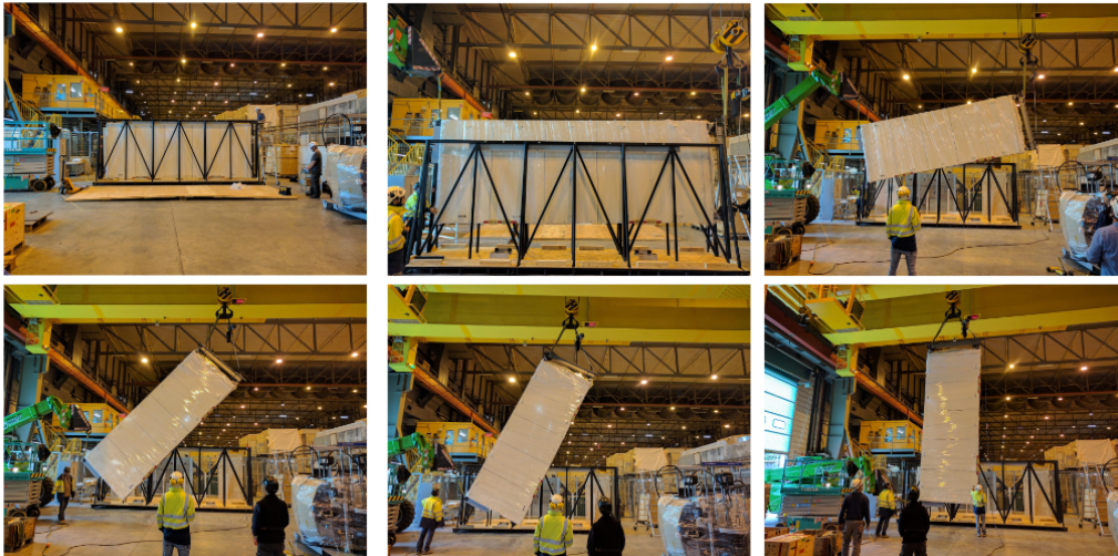
Figure 70: Arrival of an APA in EHN1 and its positioning. The upper left image shows the orientation of the APA as delivered, the lower right shows its vertical orientation when it is lowered into the material sas.
