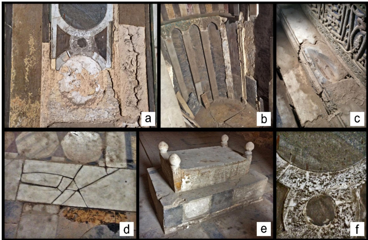
Figure 4. Different forms of deterioration in the northern mausoleum; (a) loss of material, granular disintegration, discoloration; (b) detachment of slabs; (c) fractures, erosion; (d) fractures; (e) loss of material, fractures, erosion; (f) organic staining, efflorescence.
